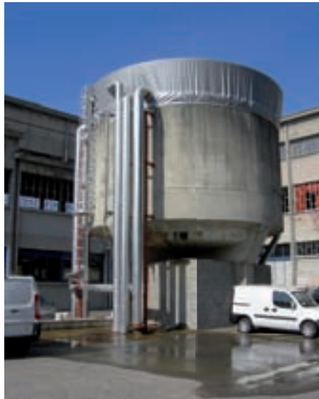
System storage tank
