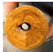
How iron contamination can affect a borehole if allowed to build up – a good reason to implement regular maintenance
