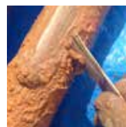
Slime on a rising main after removal from a borehole
